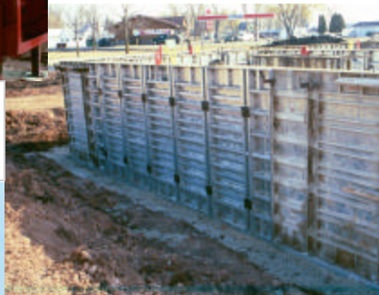
Cardinal Concrete is the 1st B.E.P. customer to have 8' high forms with just two rows of ties.
